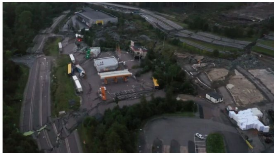
The E6 near Gothenburg was struck by a quick clay landslide on Friday night.
